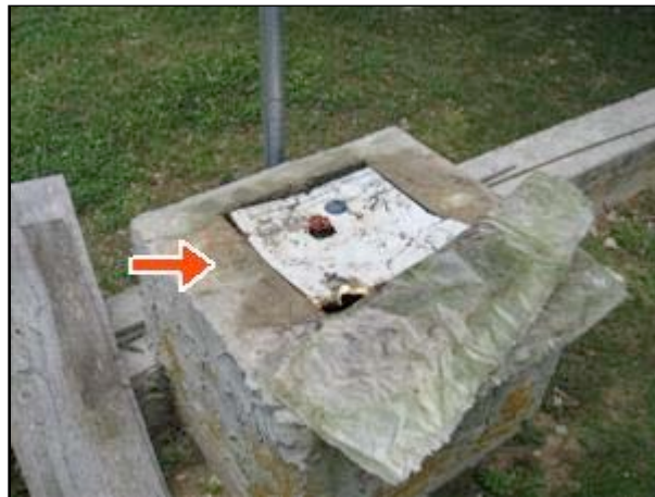
4.1 Picture 3 Well head
